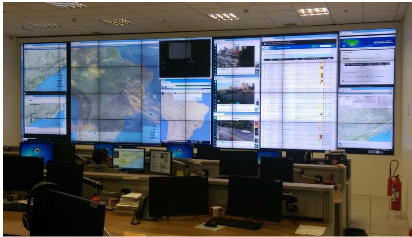
Fig. 2. Video wall in the control room of CEMADEN.
