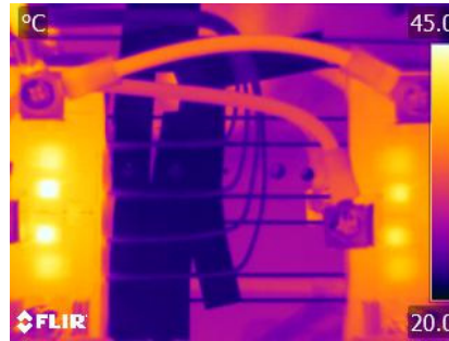
Figure 5.6: Temperature distribution measured by thermal camera
