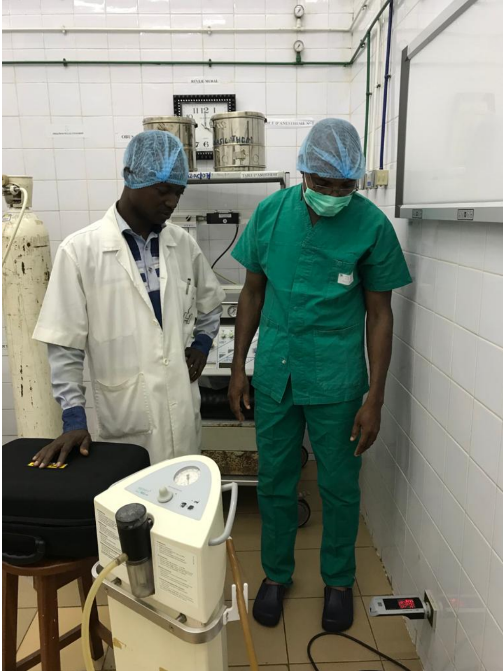
Figure 3.11: Electrical safety measurements. Details of a socket grounding that does not meet the standards, in a surgical theatre in Benin.
