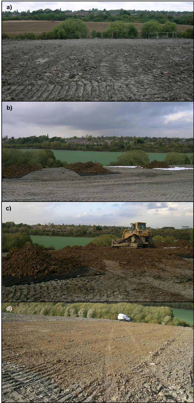
1 Fig. 1. Trial sections: a) top surface of the clay barrier; b) installation of the geosynthetic panels; 2 c) spreading the restoration soils; d) completed soil restoration.
