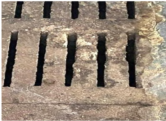
(a) Damage and corrosion of slab
