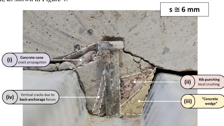
Figure 4. Damage pattern observed after testing at a slip of ca. 6 mm [10].
