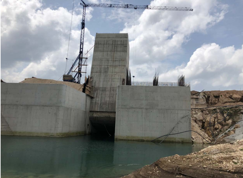
■ The construction of a derivation tunnel for HPP Dabar, the Zalomka near Biograd, the Nevesinjsko Polje, May 2022.
