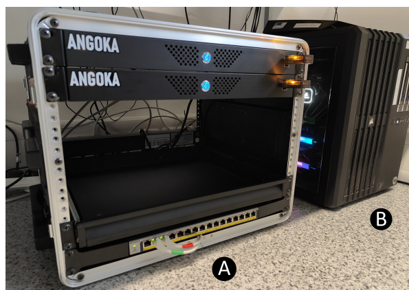
Figure 6. In this image, (A) is the Angoka V2I ZAP security system and it is installed alongside (B), which is the University of Warwick's V2I systems controller. The image was taken by AirQKD's project partner, Angoka.
