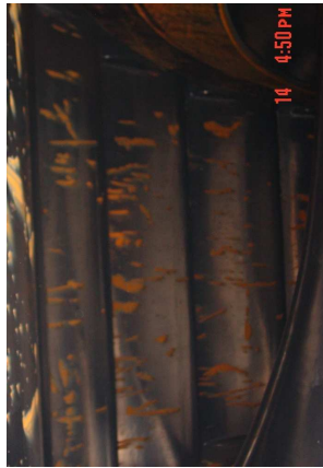
Figure 5 Damages on the lower surface on all guide vanes showing nearly the same pattern
