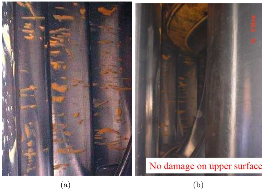
Figure 1.4: (a) Damages on the lower surfaces of all guide vanes showing nearly the same pattern; (b) No damage appeared on the upper surface [1]
