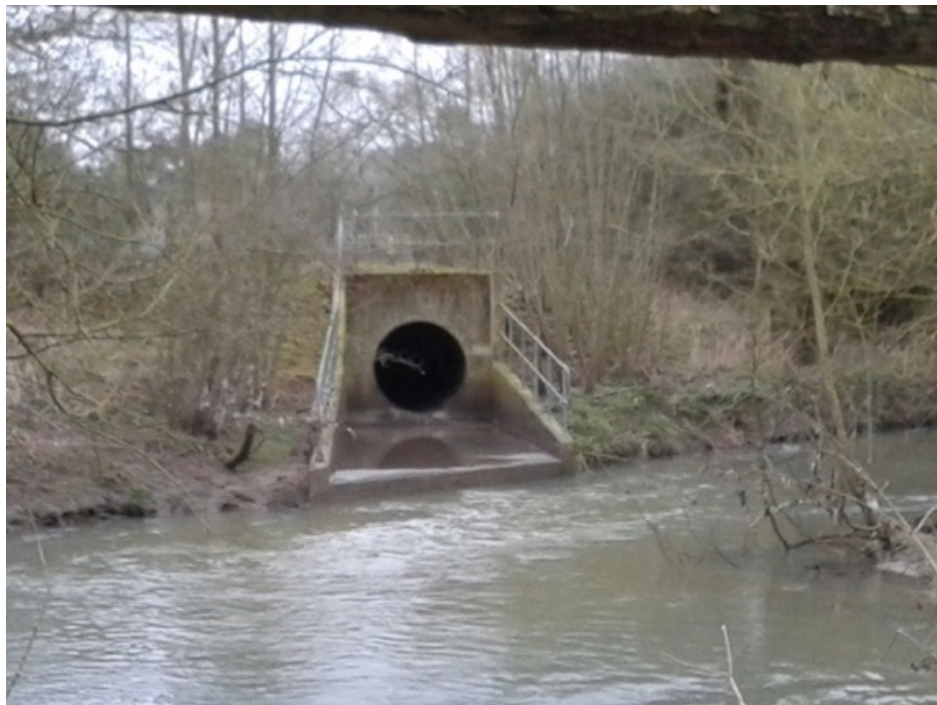
Figure 1.4 CSO release events (a) Release of untreated water from outlet pipe resulting from high level of wastewater. Dam regulates the flow of water from CSO, in times of heavy rainfall, the wastewater level increases above the threshold for the 'pass forward flow' as defined by the EA and untreated wastewater is released directly in to receiving water bodies. (b) photograph of one of the CSO release sites from the Finham WWTP.
